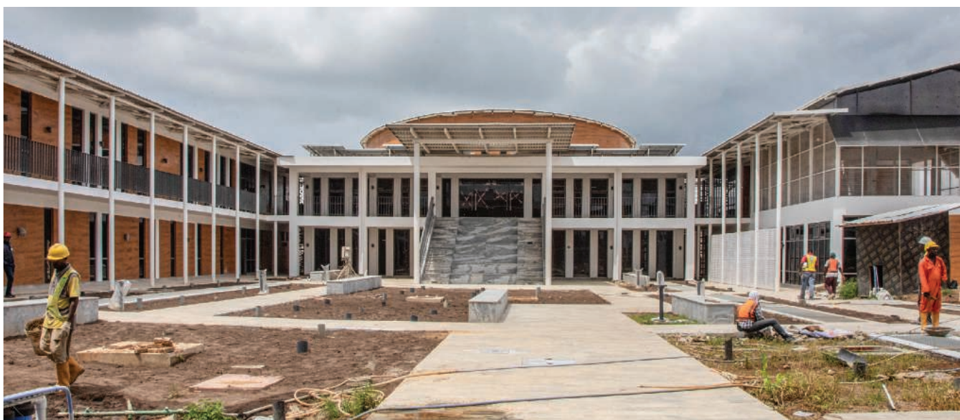
Construction workers in late April put finishing touches on a new, $10 million sequencing center in Ede, Nigeria, which includes a conference room, dorms, and classrooms.
