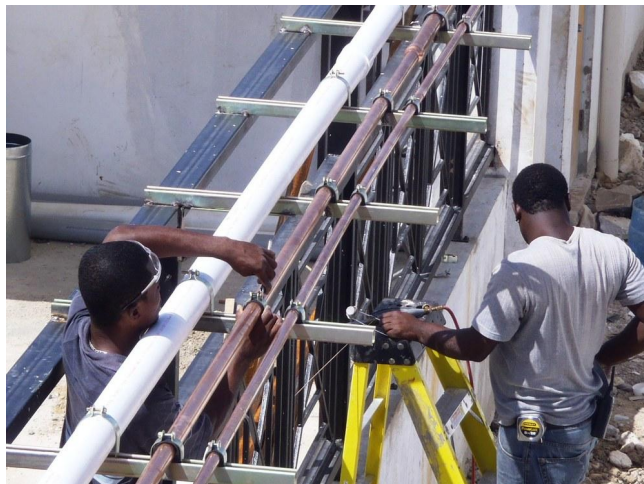
Figure 5a: MGPS running above ground*
