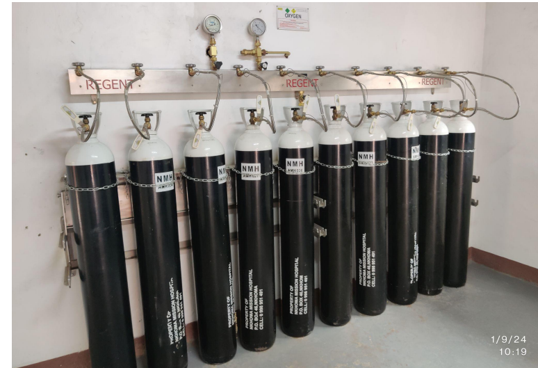
Figure 2b: Cylinder supply manifold restrained with chains
