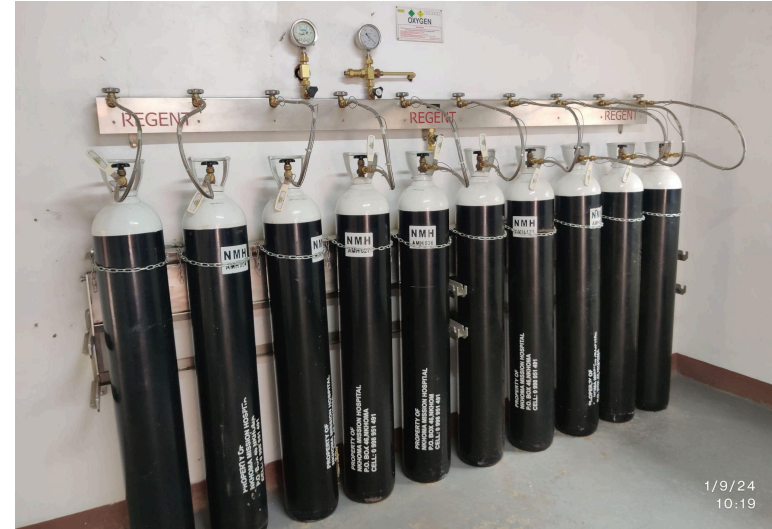
Figure 2b: Cylinder supply manifold restrained with chains
