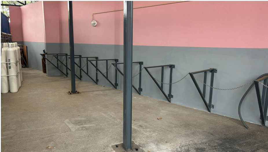
Figure 4a: Cylinder storage area with racks and chains (no cylinders pictured)
