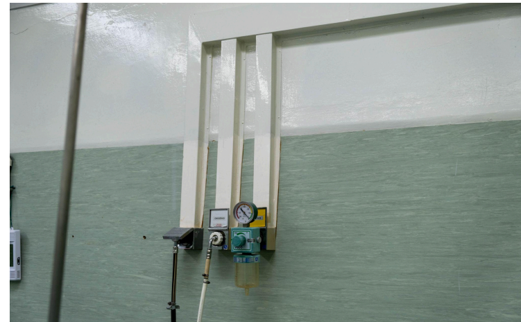
Figure 3b: Wall-mounted oxygen outlet (supplied by cylinder manifold or MGPS direct from the oxygen plant)
