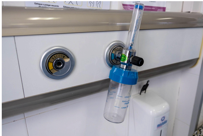
Figure 3a: Wall-mounted oxygen outlet (supplied by cylinder manifold or MGPS direct from the oxygen plant)
