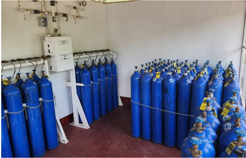
Figure 2a: Cylinder supply manifold and storage restrained with chains
